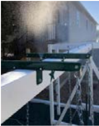
Swing Beam Misting System
